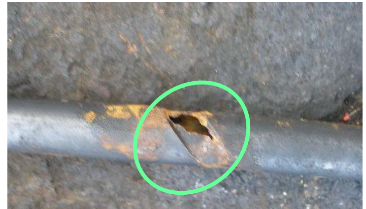
Tube damage from flow-induced vibrations
