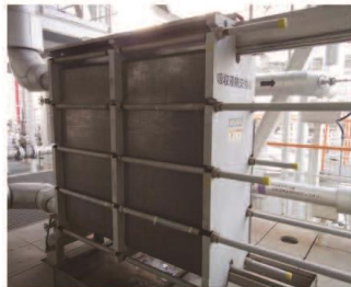
CO 2 recovery, desulfurization plant solution heat exchange
