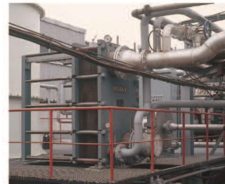
Solvent recovery, exhaust gas cooling
