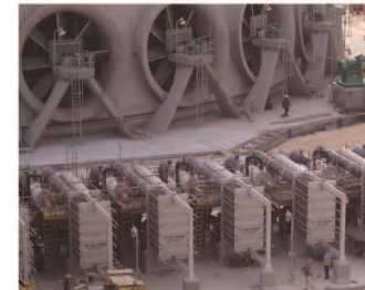
Central cooling system
