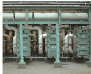
Sulfuric acid, electrolytic plating cooling
