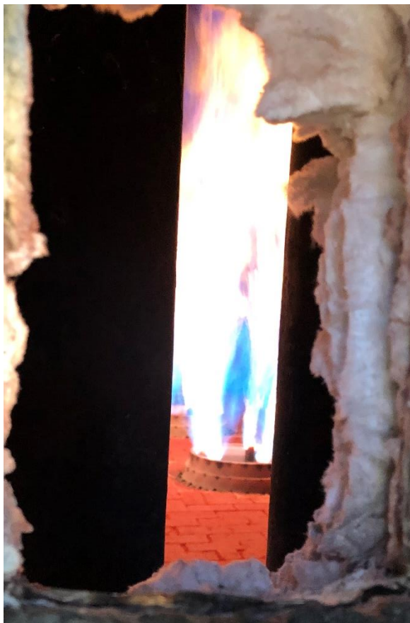
Floor burner flame
