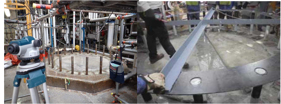
Padding and anchor bolt inspection : To Ensure bolt arrangement and pad leveling
