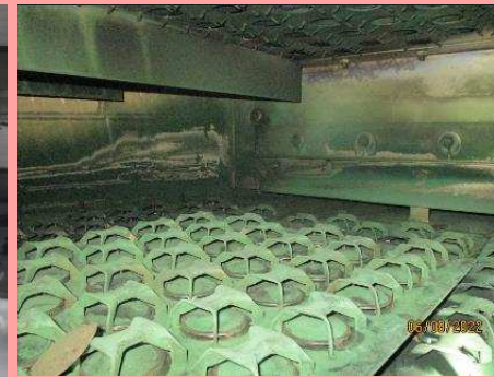
2 Green corrosion product
