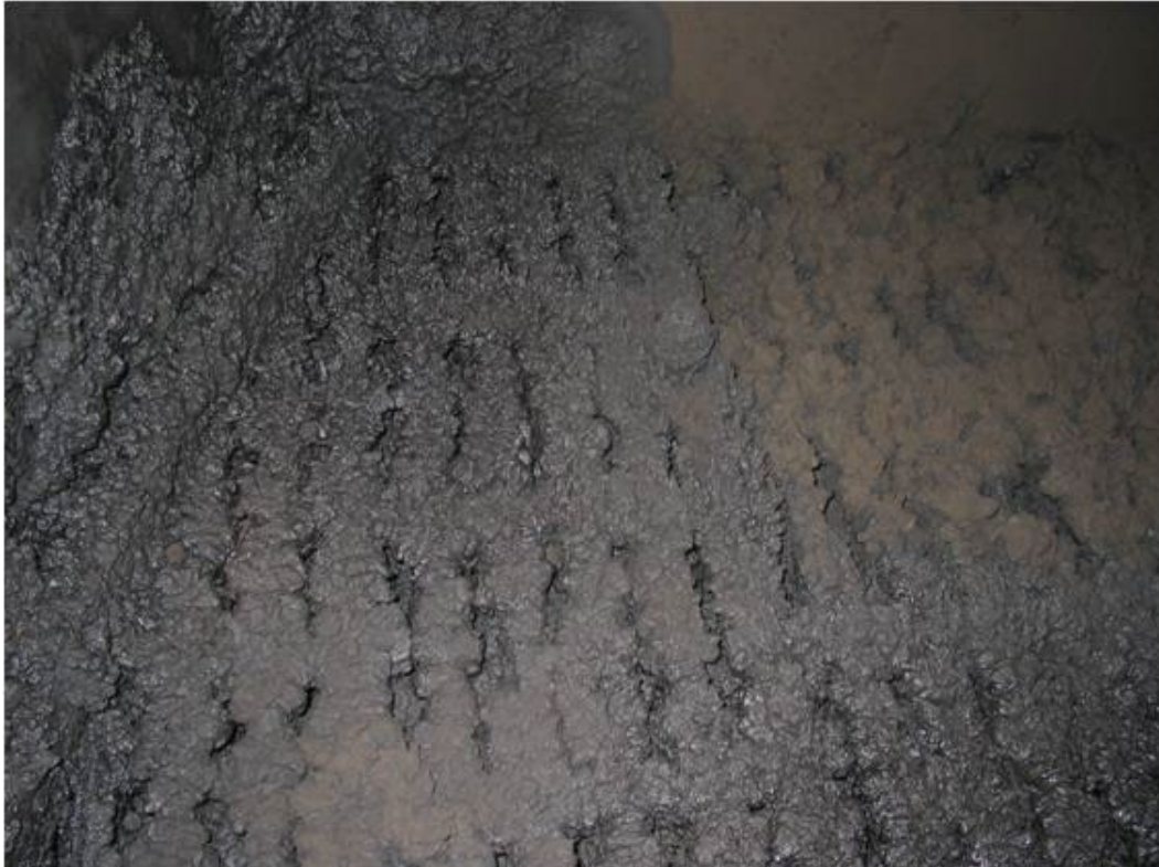
SEVERE COKING OF GRID PACKING
