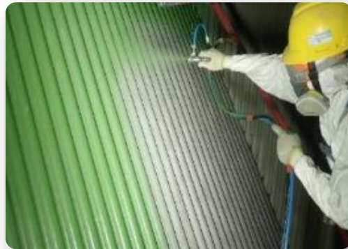
WATER WALL TUBE
