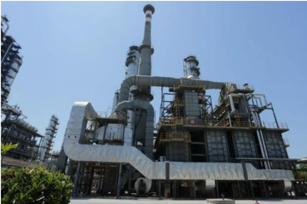
Refinery H CDU Heater
